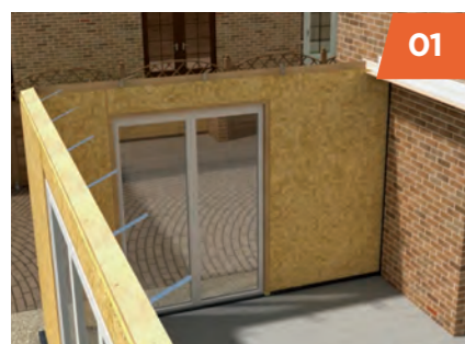
01 Structural ringbeam is sealed and secured to the top of the Kingspan TEK® wall structure.
