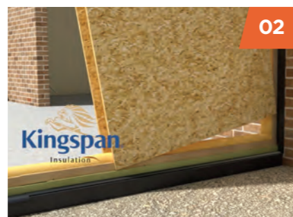
02 Wall and sole plates installed ready to receive the Kingspan TEK® panels.
