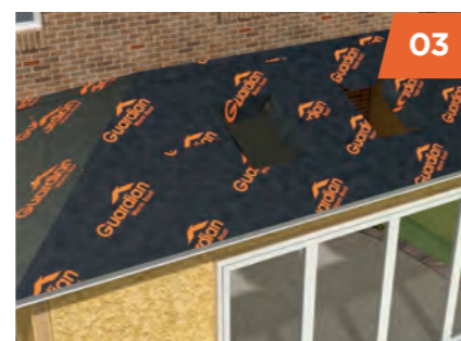
03 Breathable waterproof membrane is laid over the plywood and secured in place.
