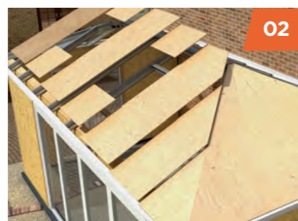
02 The aluminium roof structure is secured to the ring-beam and exterior grade ply-board is fixed.
